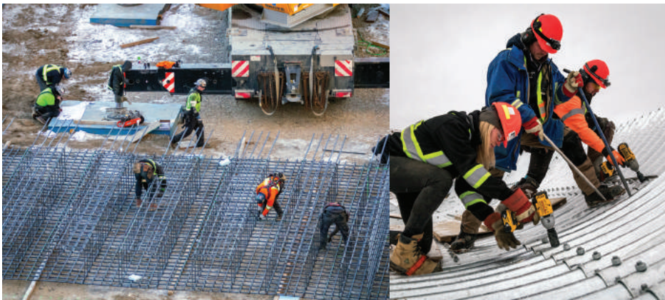
/ Yukoners at Work preparing rebar for the Primary Crusher, and installing the CSP tunnel at the Coarse Ore Stockpile.
