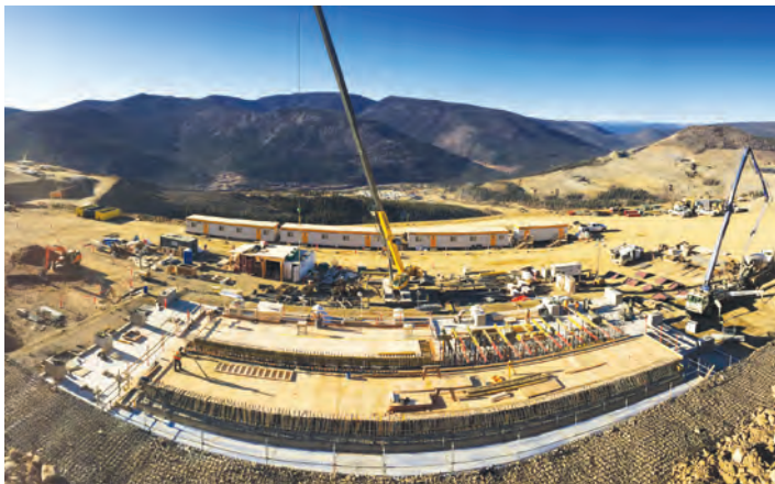
Construction of the Secondary Crusher with a view of the camp in the centre background.
