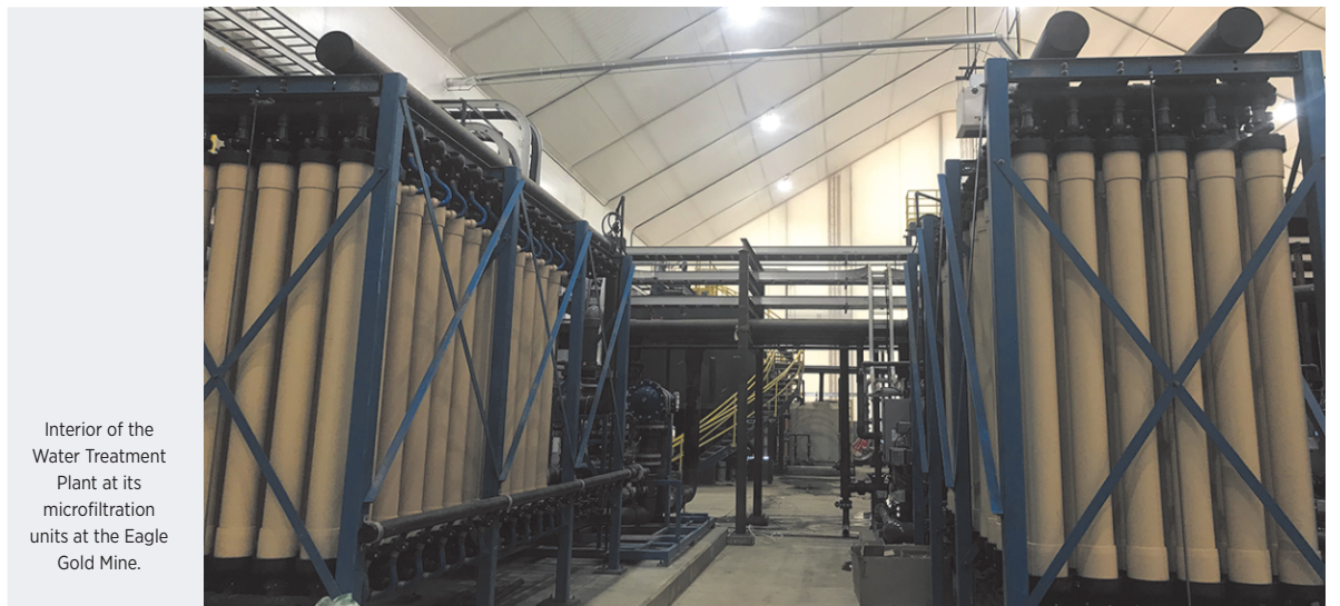
Victoria Gold's Water Treatment Plant at the Eagle Gold Mine.
